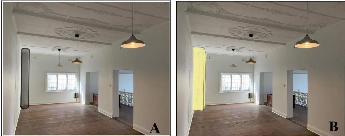
Figure 8. The steel pipe screwpile in the left corner (A). Image B shows the temporary cover through which the pile is drilled.
